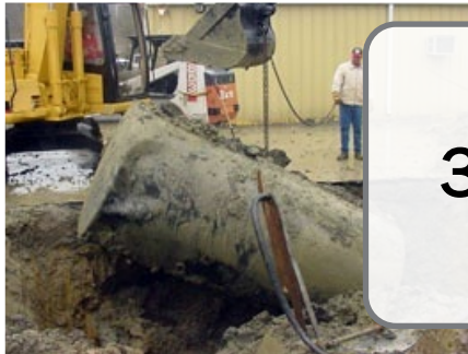
Underground Storage Tanks
